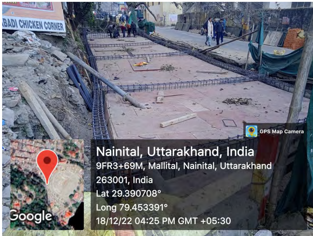
The trunk storm water drain, flowing into the Naini Lake, being concretized and covered with thick slabs, in Mallital.
